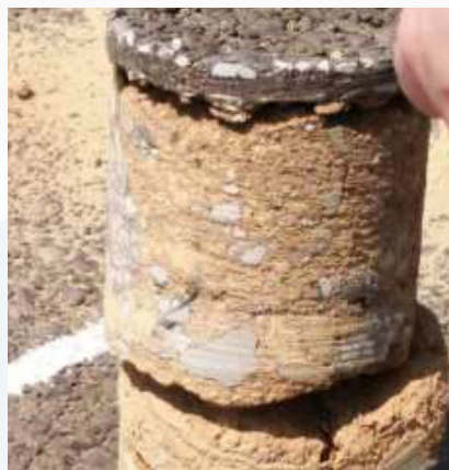
Drilled core showing the double seal, 150mm NME 4 base-layer (1.5% NME) and 150mm sub-base layer (1.0% NME). (NB: NO CEMENT!)
