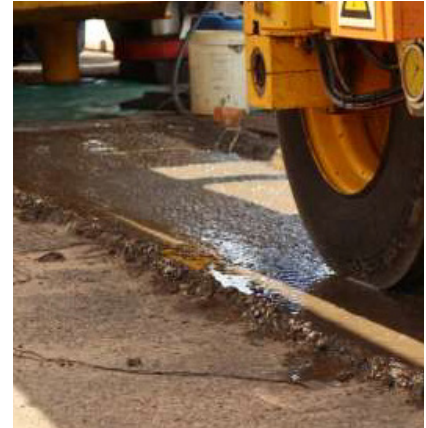
(8 January 2019) Testing at a dual wheel load of 80 kN with water applied continuously on the surfacing and to a depth of 500 mm through holes next to the test section.
