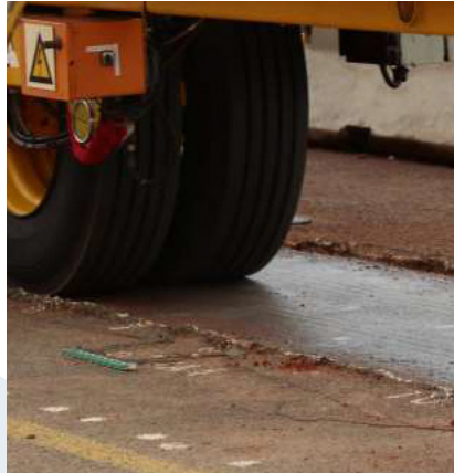
(26 November 2018) Wheel load at 80 kN (double normal). No deformation or damage to base or sub-base (seal pushed aside due to spillage of hydraulic oil from a burst pipe on the HVS) – 3 Million E80s applied to test section.
