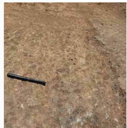
Condition of the exposed base-layer at the end of the test after removal of the surfacing with a hammer and chisel.
